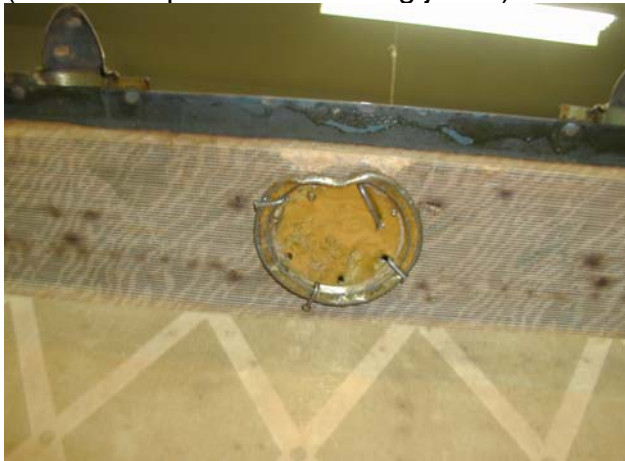
Interior of the lock – previous repair (The brass plate is a canning jar lid)
